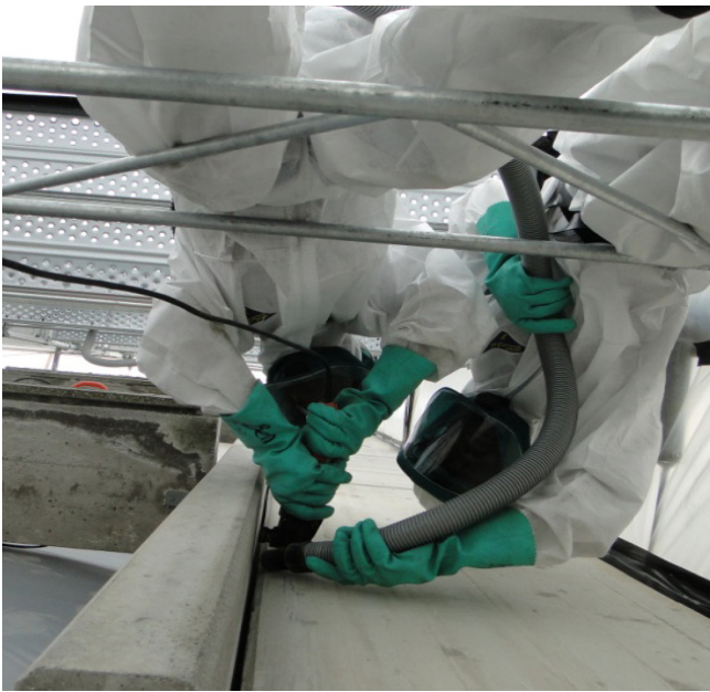
Figure 3: Removal of PCBs caulks in a Clean up Zone in a residential building (Source ETI)
