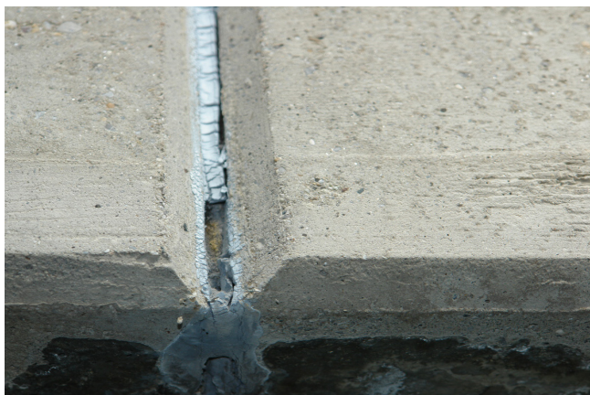
Figure 1: PCB containing caulk (sealant) in façade (Source: ETI)
