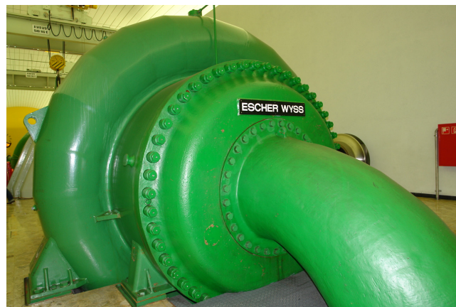
Figure 2: PCB containing anti-corrosion coating on a turbine (Source ETI)
