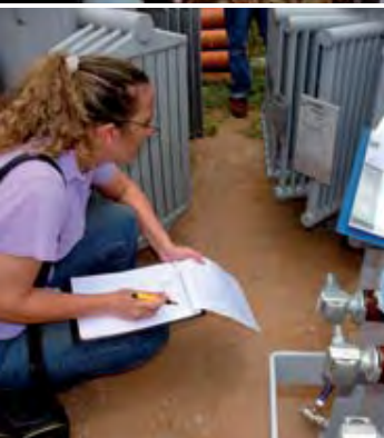
Inventory of transformers in Paraguay
