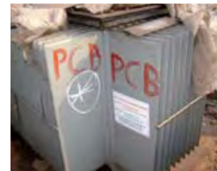
Electrical transformer containing PCB (PCB level > 500 ppm)
