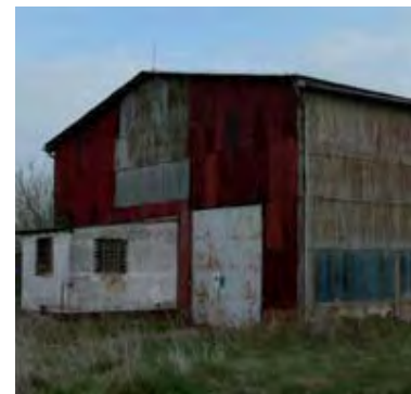
Two storage sites in the Czech Republic, where PCB are not stored securely
