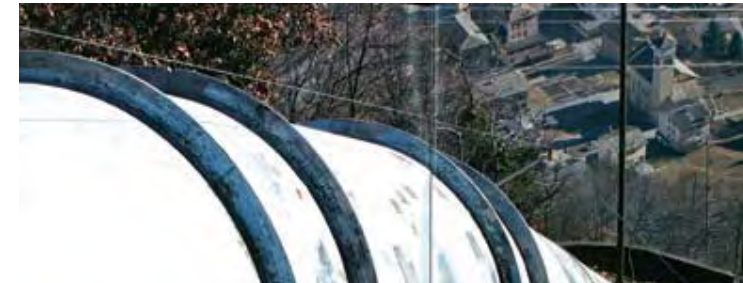
Pressure water pipeline with PCB coating inside and outside
