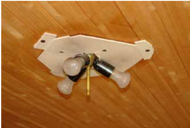
Figure 3: Asbestos cardboard under lamp (Source: ETI [4])
